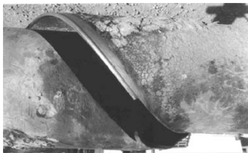
Fig. 9 SOHIC failure of NPS 16 spiral-welded linepipe (Canada 1979 failure; courtesy M. Hay/Shell Canada)
